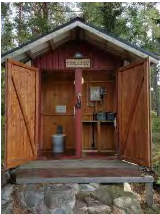
Picture 51. Northern pier: There was space for the solar power equipment in the existing toilet building. © Per-Olov Persson
