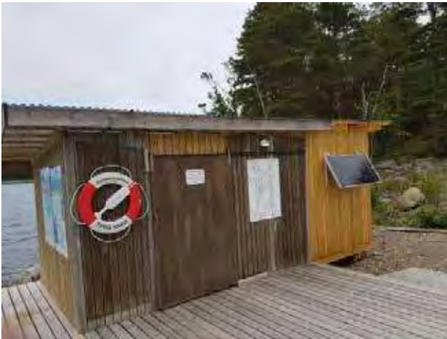
Picture 54. Southern pier: The existing waste sorting building is being expanded with space for a solar panel and equipment room. © Per-Olov Persson
