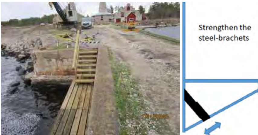
Pictures 39 and 40. Part of the renewed walking decks and new stairs up to quya from the walking deck and illustration of the strengthening measure. © Leif Ortman
