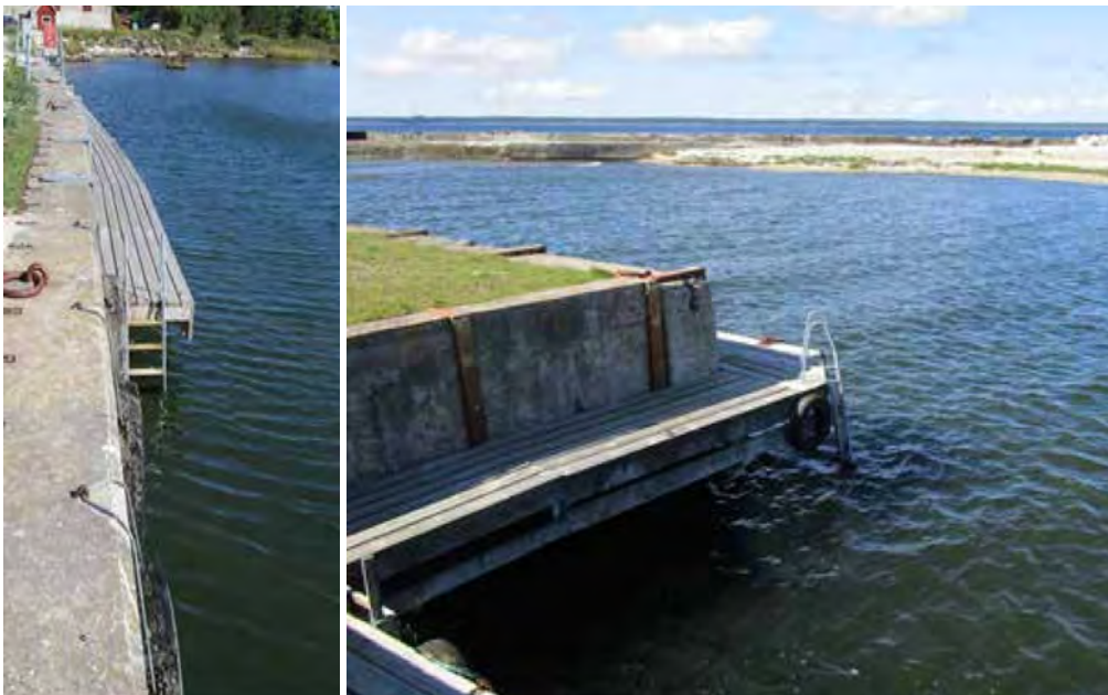
Pictures 41 and 42. The safety-ladders from water to the walking deck. © Leif Ortman
