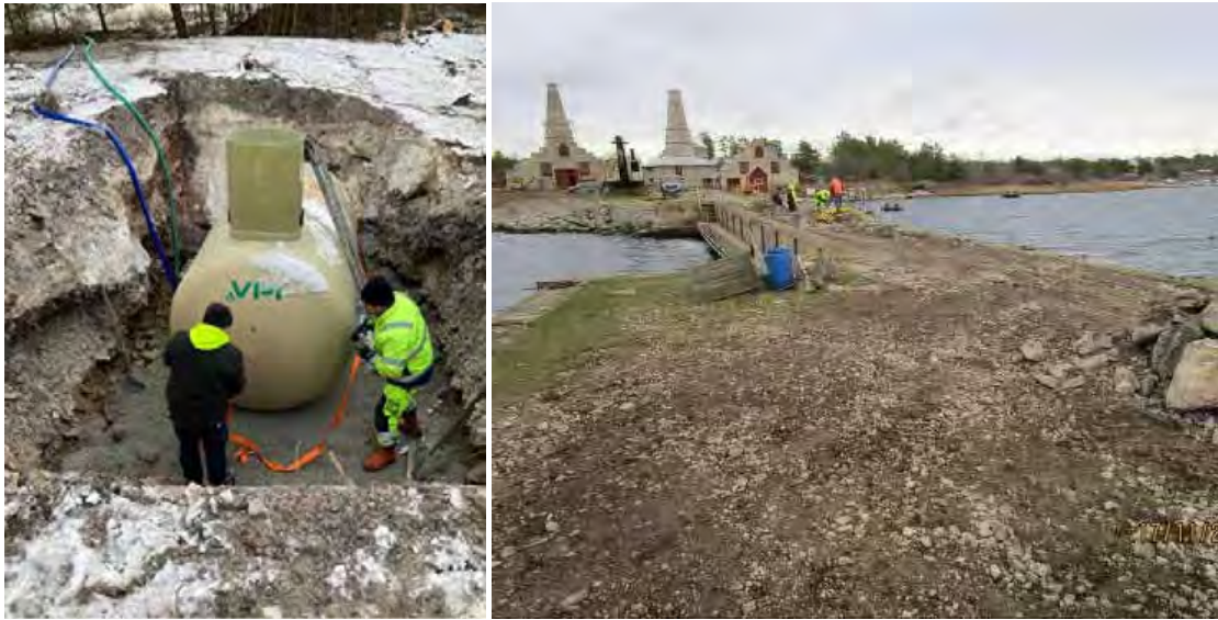
Pictures 45. Installing the septic waste tank and picture 46. Excavation work on quay. © Leif Ortman
