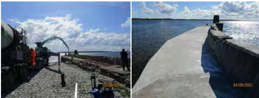
Pictures 47 and 48. ESB.2 Concrete casting ongoing and results for breakwater. © Leif Ortman
