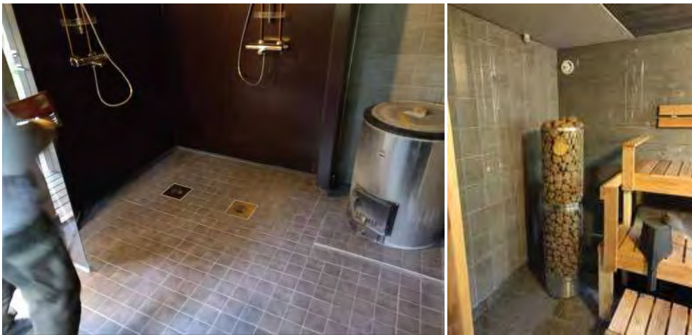
Pictures 5 and 6. Renovated shower and heated rooms of the Beach/log sauna building. © Teemu Heikkinen
