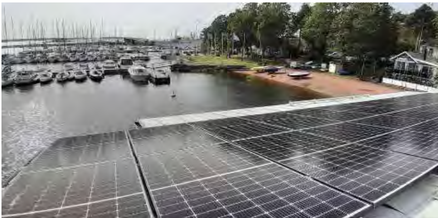
Picture 19. Sapokka's new solar power plant in August 2021. © Jussi Sutela
