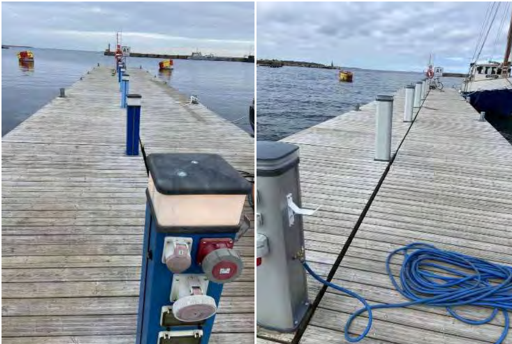
Pictures 57 and 58. Old and new service stands in one of the piers in Lennusadam. © Lauri Väinsalu
